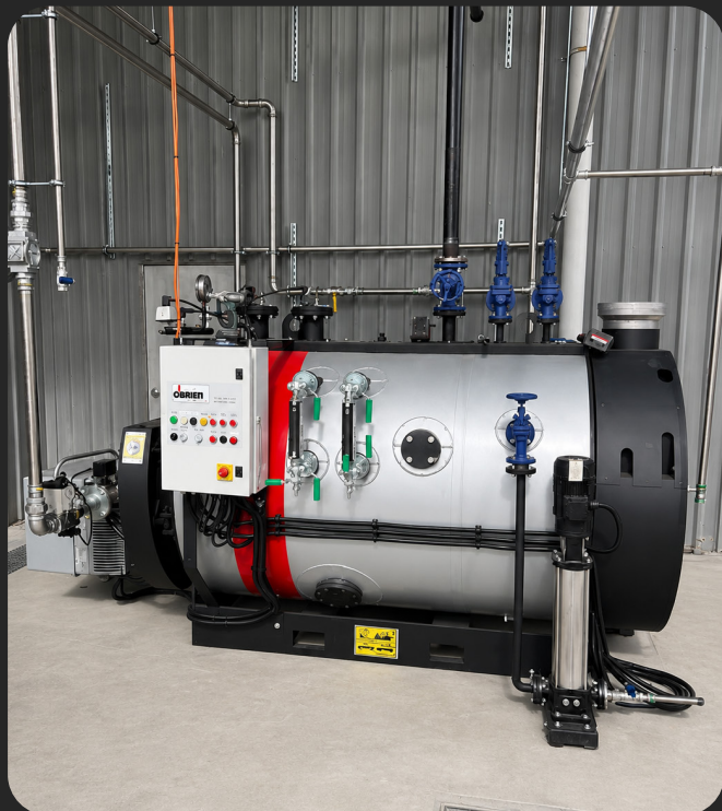
500KW OBYONE800 Steam Boiler M&KH Trading, NSW
