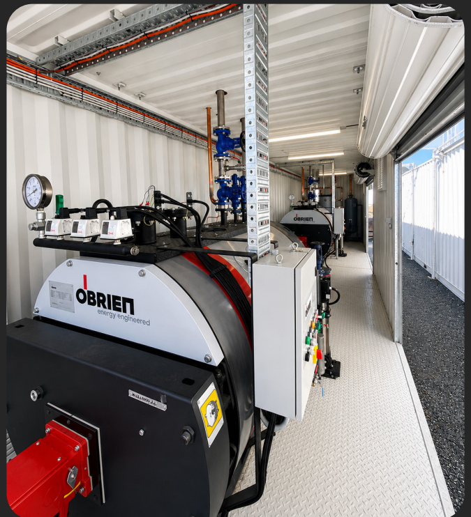
4000kW OBYONE3P-6000 Steam Boiler, Orica 136 Turpentine St, Blackwater 4717, QLD
